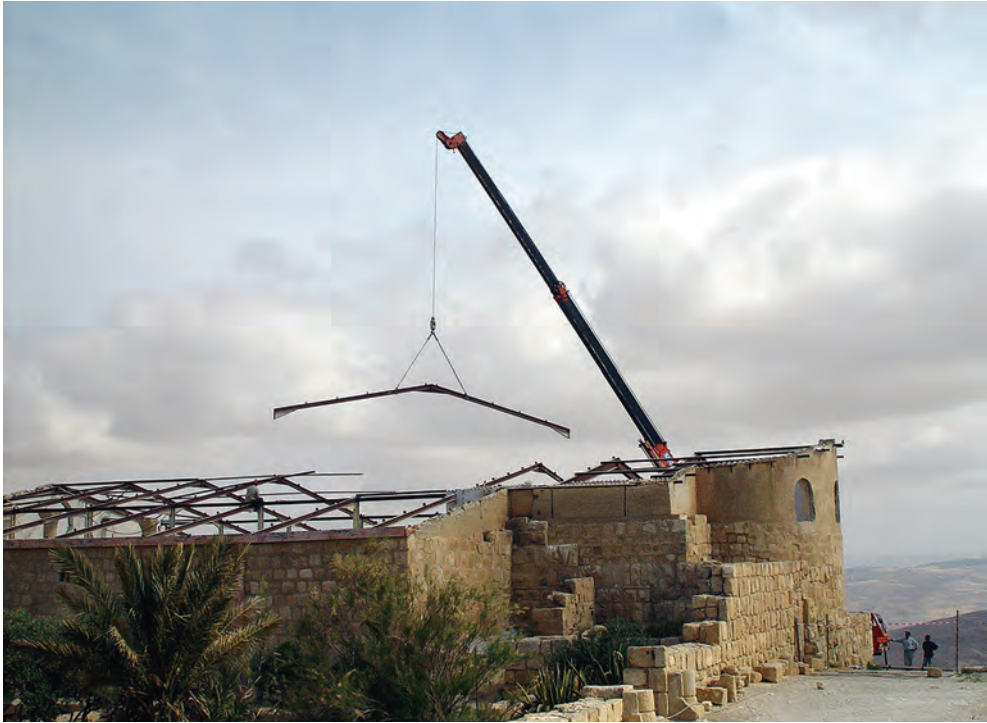
Fig. 5. The dismantling of the iron structure of the old shelter, April 2008 (© C. Pappalardo)
