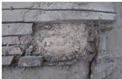
Fig. 5. The remnants of the original mortar layers photographed with oblique lighting (photo: Brigitta Maria Kürtösi)
