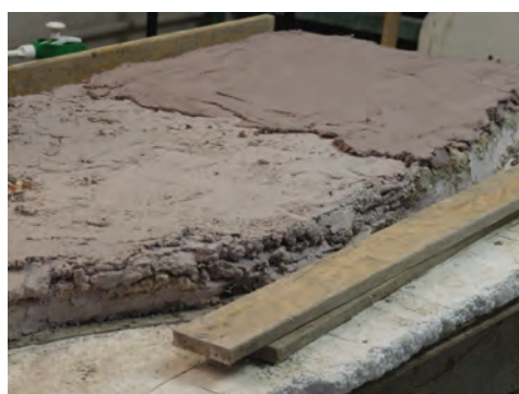
Fig. 12. The leveling of the backside of the mosaic was made by the lightweight lime-based mortar (Photo: Brigitta Maria Kürtösi)
