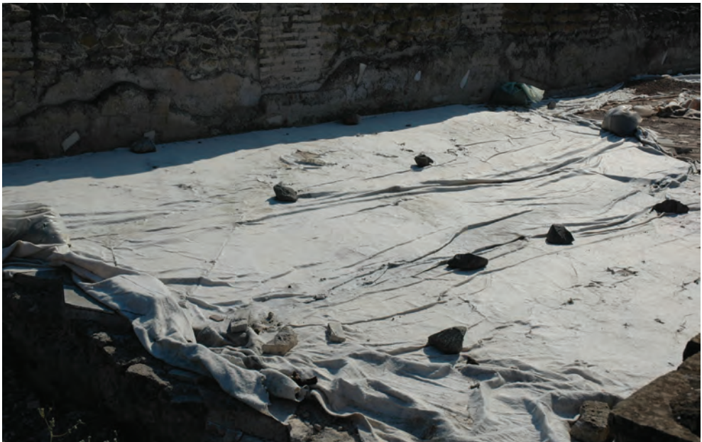
Fig. 2. Covering mosaic floors with nonwoven fabric, Villa dei Quintilii, Rome (photo: A. Lugari)
