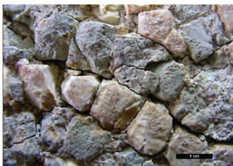
Fig. 8. Rounded and cracked tesserae after the loss of edges and corners
