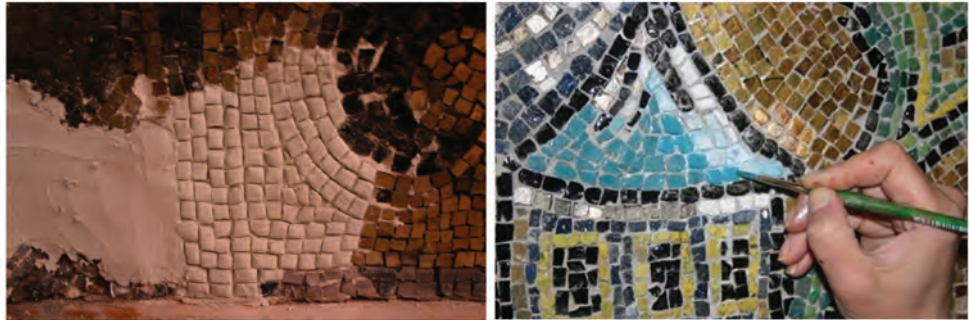
Fig. 9. Interventions-refilling of the lacunae and colouring (photo: M. Jbaee 2008, by permission of DGAM, Syria)
