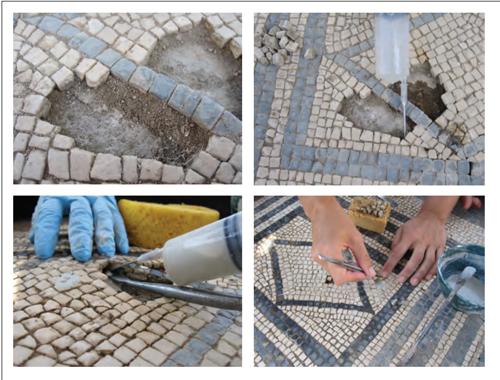
Fig. 11. Conservation work from 2011 on a black and white mosaic from Domus 1 : application of a biocide, setting bulged areas with natural mortars and re-laying detached tesserae (photo: Sílvia Llobet)
