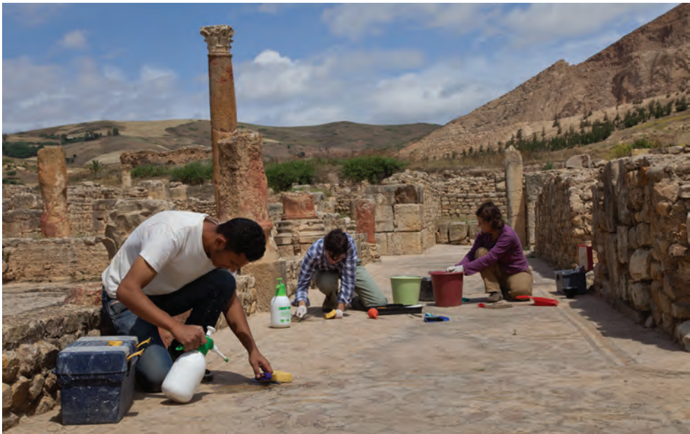
Fig. 1. Recently trained INP technicians with periodic GCI supervision conserving the mosaics of the Maison de la Chasse (photo: Scott S. Warren © 2011 The J. Paul Getty Trust)
