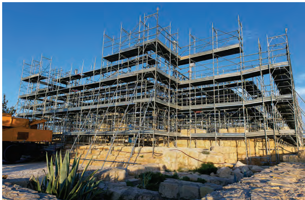
Fig. 6. The scaffolding on the Memorial's perimeter for the building of the new shelter, March 2010 (© C. Pappalardo)
