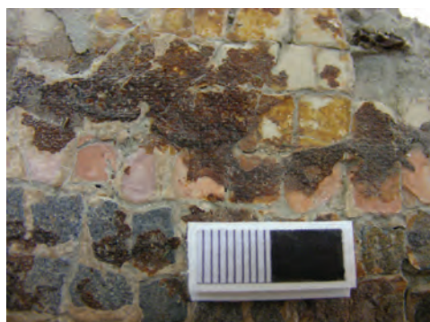
Fig. 6. Deteriorated remains of rubber glue
