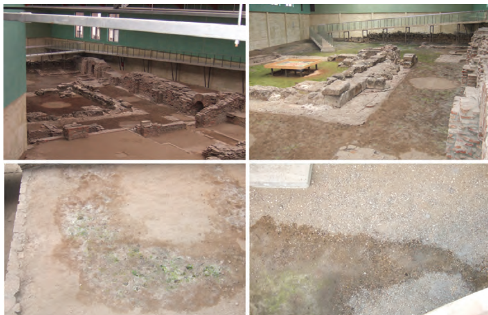
Fig. 13. Examples of rising damp (photos: N. Smiciklas, Institute for the Protection of Cultural Monuments of Serbia, Belgrade)
