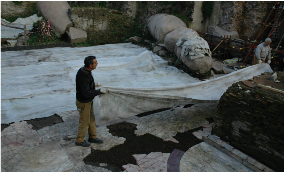
Fig. 4. Daily covering with nonwoven fabric, Forum of Peace, Imperial Fora, Rome (photo: A. Lugari)
