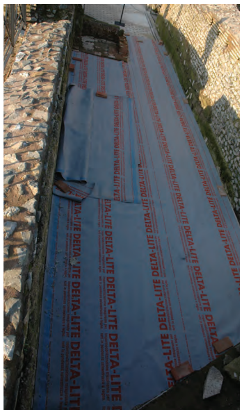
Fig. 9. Covering with a 'single' sheet of Delta-Lite fabric, Villa dei Quintilii, Rome (photo: A. Lugari)
