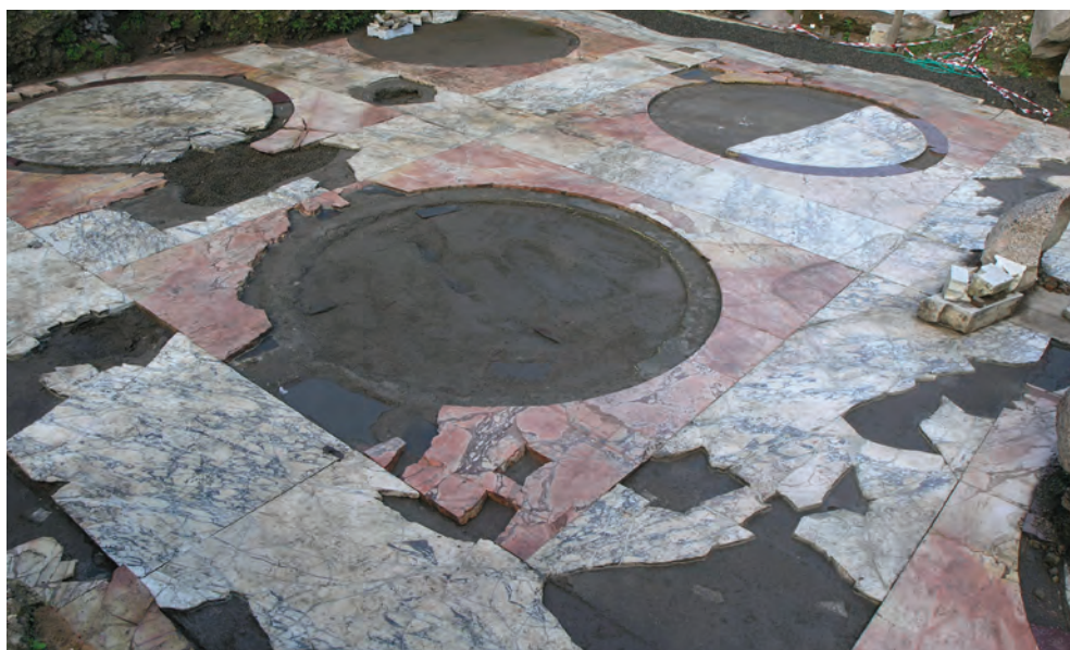
Fig. 7. Condition after one year of covering with Delta-Lite fabric, Forum of Peace, Imperial Fora, Rome (photo: A. Lugari)
