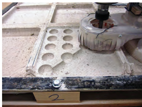
Fig. 4 Initial cutting patterns to mill concrete within steel grids (photo: Yale University Art Gallery)
