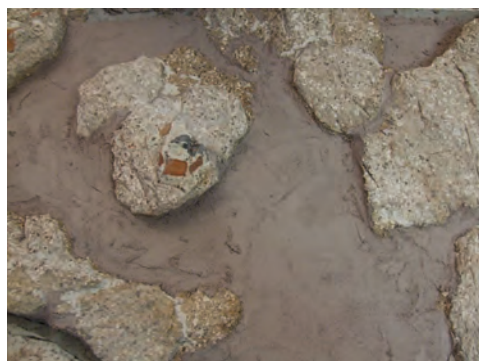
Fig. 11. The leveling of the backside of the mosaic was made by the lightweight lime-based mortar (Photo: Brigitta Maria Kürtösi)
