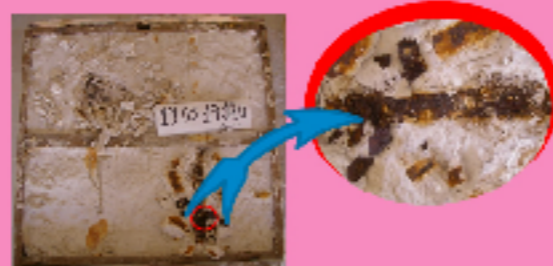
corrosion of slats metal
