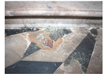
Altar right side: alongside the building structures, moisture and salts cause visible damage to the very thin tarsia slabs. Under them, the rosin mixture is often dusty and poorly conserved.
