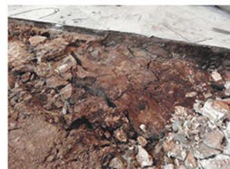
Main altar: the rosin mixture employed for the slabs settlement was extremely fragmented and dusty.
