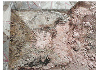
Sanctuary area: use of different kinds of mortars, employed side by side with no differentiation, to settle the marble slabs.
